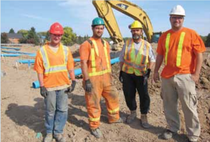
One of the Alfred Beam excavating crews is working on servicing a new subdivision in Niagara-on-the-Lake. Pictured from left are James Poirier, Pat Murphy, Jeffrey Bateman and foreman Shawn Schertzing.
